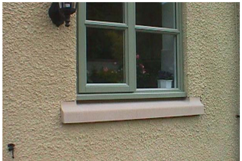
Area of window, after application of Mendrend
