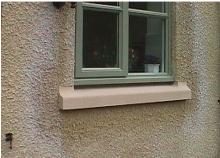
Area of window prior to the application of Mendrend
