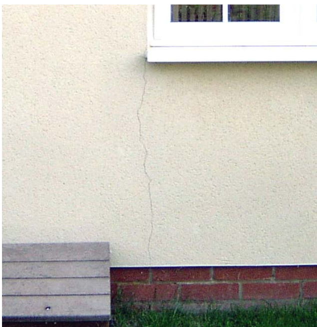
Example of cracking
